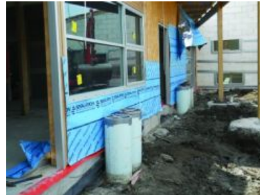
The intake ducts, taped off and yet to be finished off with cowls, adjacent to the school's external walls
